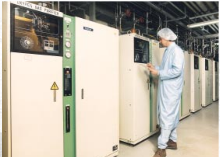
Additional gas purifier
